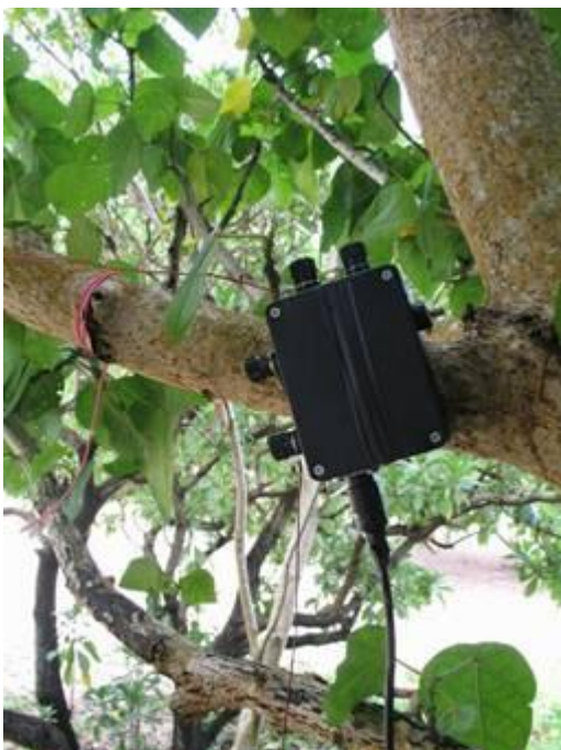
Fig. 12. Remote end of the Beverage control box
